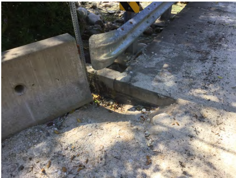
Fill erosion upstream right approach
