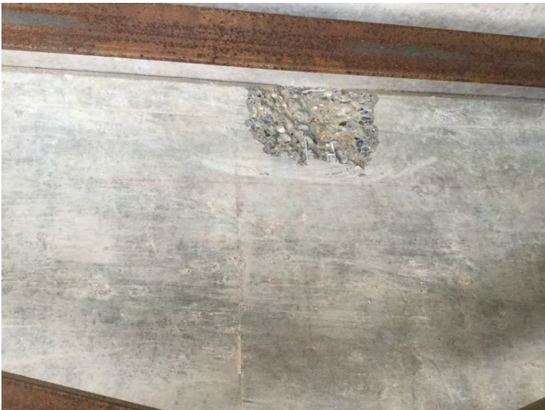
Minor damage to left bank approach ballast wall
